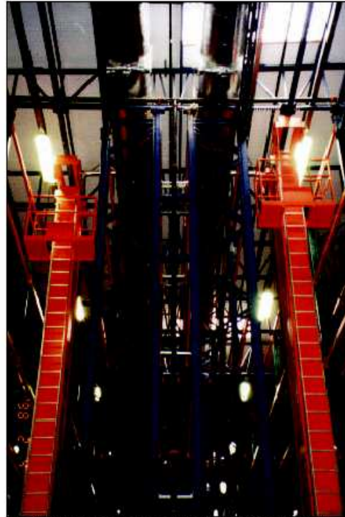
The ductwork and nozzles are contained within the roof steelwork and do not interfere with the automatic craneage and handling systems.
